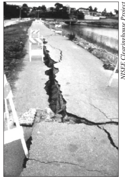
Figure 35 - Lateral Spreading, Loma Prieta Earthquake, October 17, 1989. Lateral spreading damaged levee road along the San Lorenzo River.
