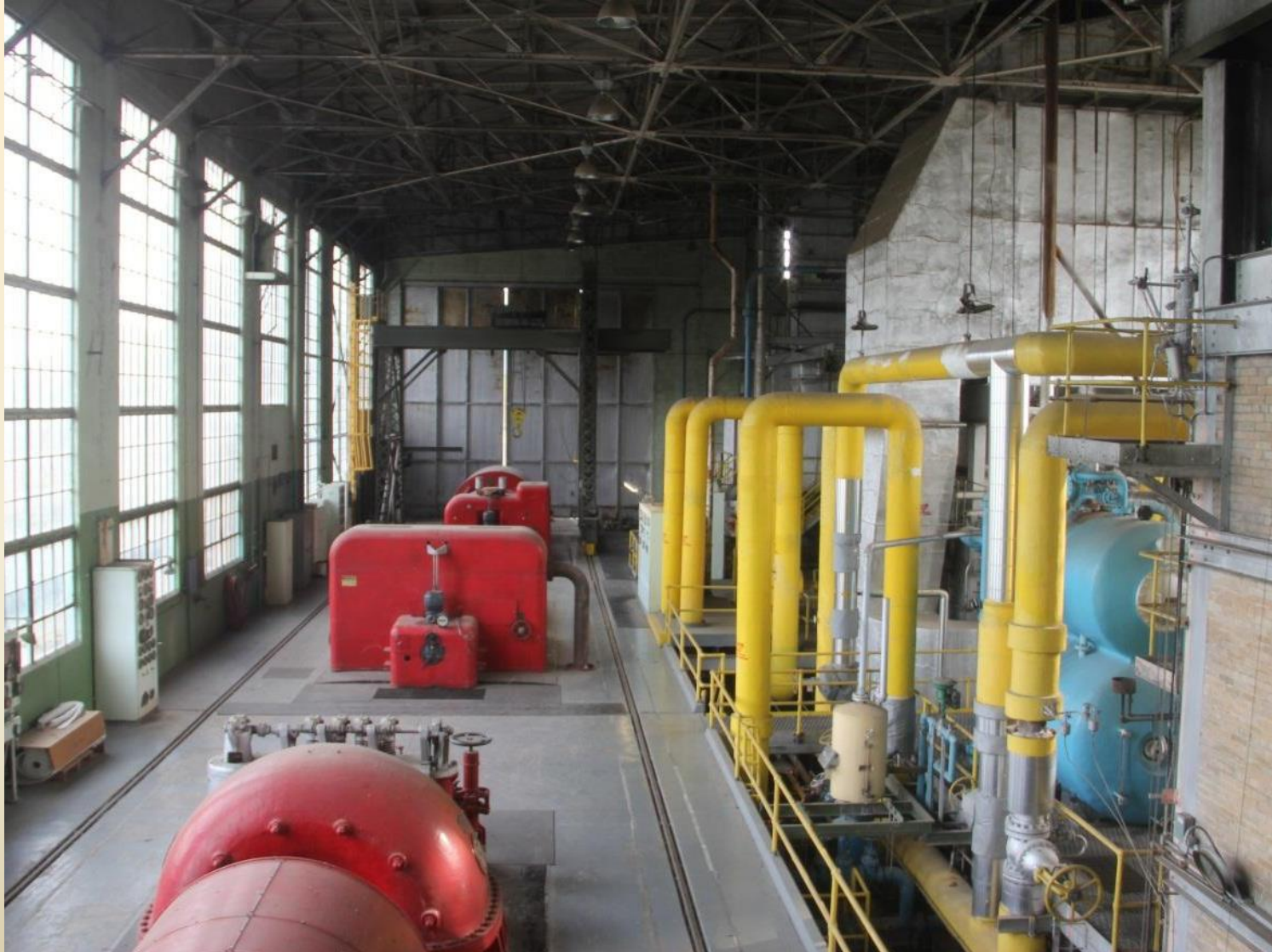
Turbine and boiler #1 in foreground.
