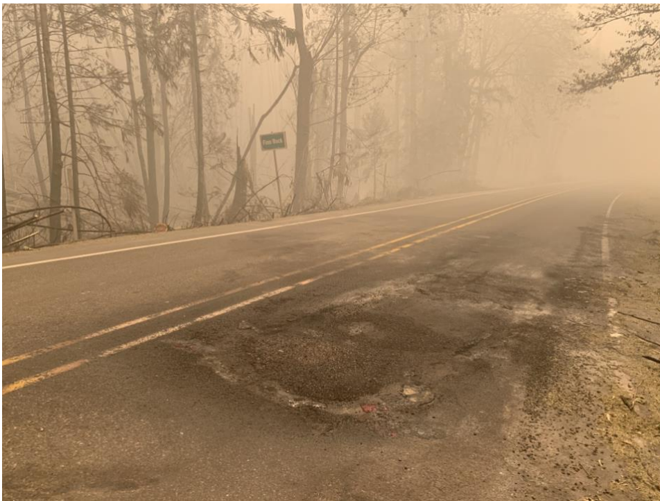
Road damage on Highway OR 126 during the Holiday Farm Fire in September 2020. Courtesy of Oregon Department of Transportation.
