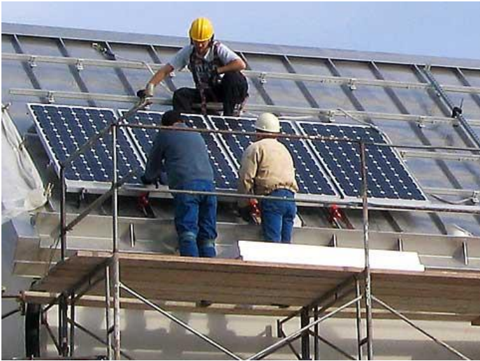
Solar panels are installed at St. Vincent de Paul in Eugene. EWEB photo.
