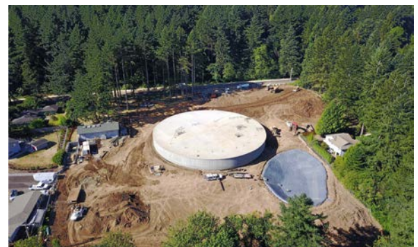
Examples of tank construction in Mt. Vernon WA (6 MG) and West linn OR (4 MV)
