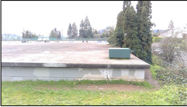
Figure 3.1-3. College Hill Reservoir 603 ( foreground ), with College Hill Reservoir 607 partially visible ( back ); view south.
