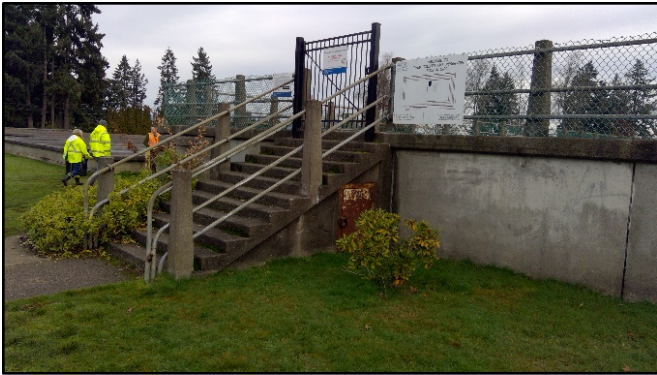
Figure 3.3-3. College Hill Reservoir 607, stairway on north end of west face; view northeast.
