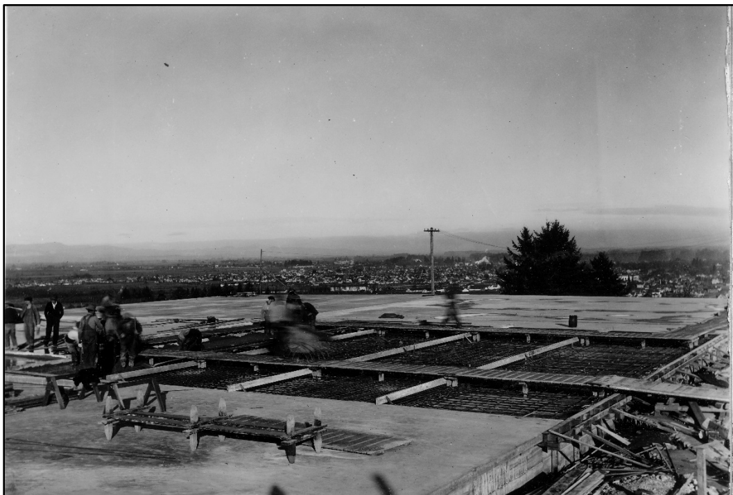
Figure 3.1-7. College Hill Reservoir 603 cover, view showing No. 5 panel during placing of concrete. Photo by W. J. Moore, November 21, 1933. Image No. 1245, courtesy of EWEB.
