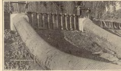
EIGHT-FOOT DIAMETER WOOD-STAVE PIPE PENSTOCKS Banded with 3/4-INCH STEEL; EUGENE, ORE., HYDROELECTRIC PLANT
