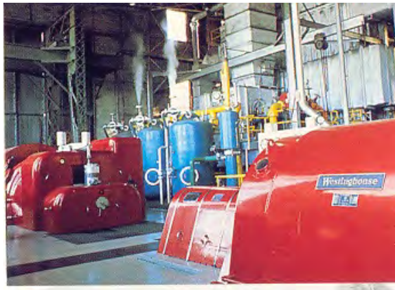
Figure 2-127 Steam Plant Turbines (red) - 1985
