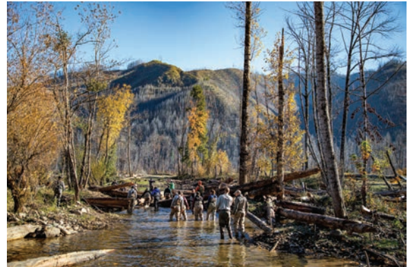
Sustainability + Resilience in Action: EWEB and partners are restoring the natural functions of Finn Rock Reach along the McKenzie River, protecting natural resources and improving long-term drinking water quality.
